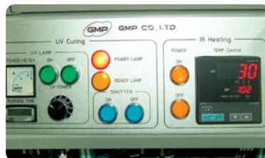
▶ UV Control Panel
